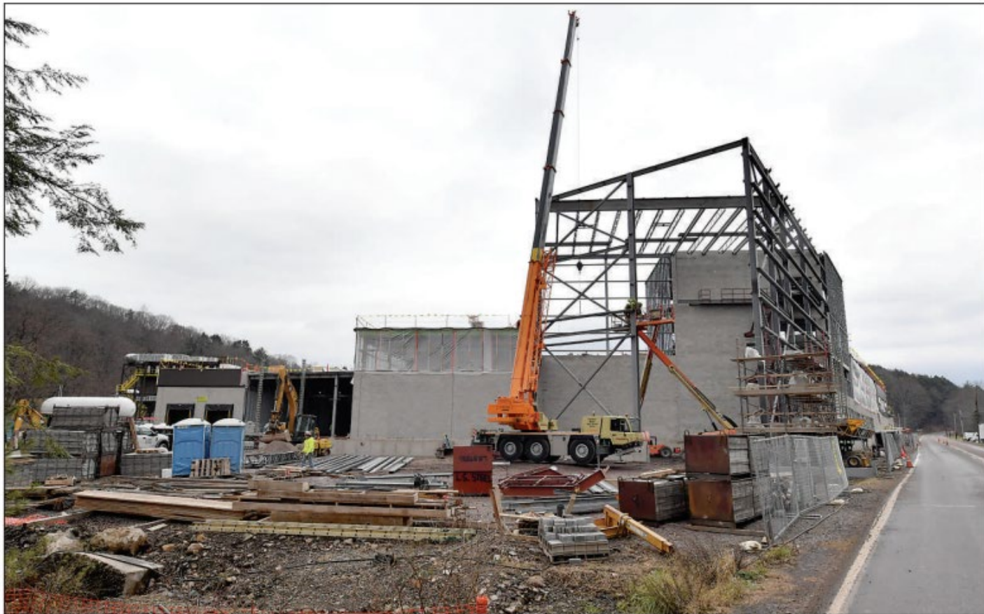
WORKERS stand steel Monday as the addition to the Benton Foundry progresses. It is located in Sugarloaf Township.
